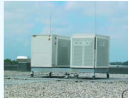
The external central heat pump installed at Nic. Oud Direct Mail, Holland
